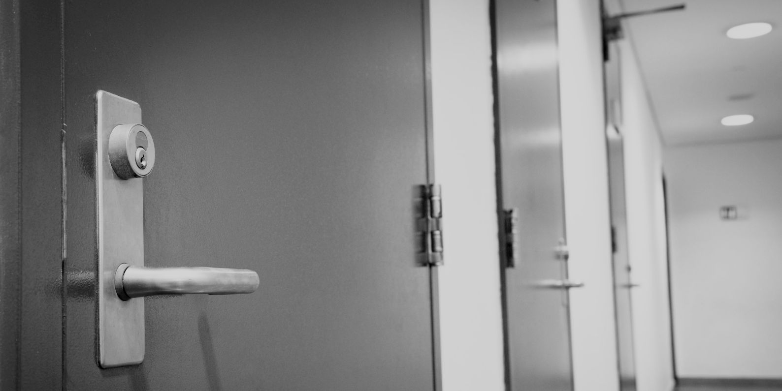
Fitzpatrick Fire doors installed at Beirut City Center
