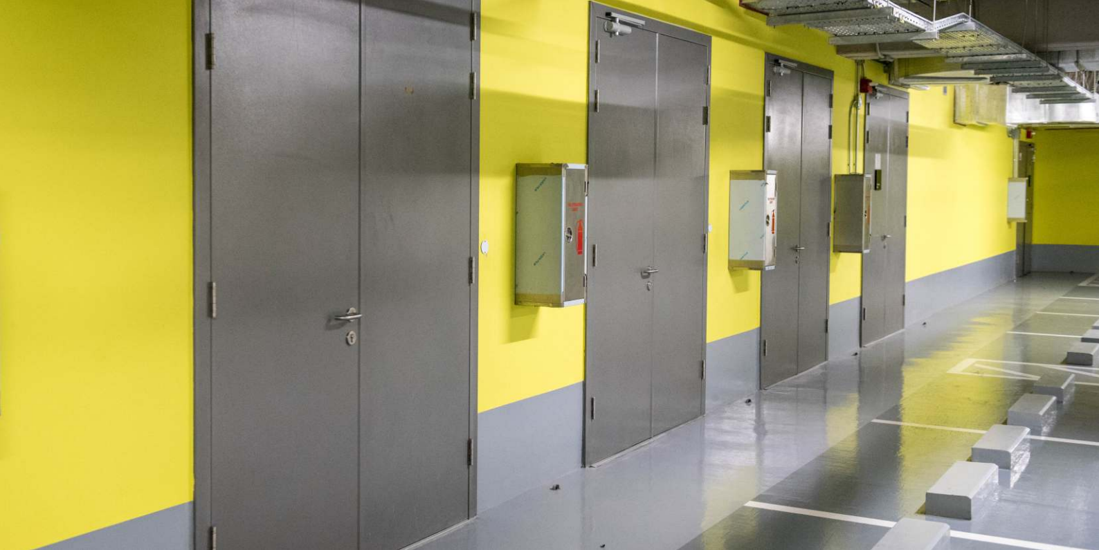
Fitzpatrick fire rated doors installed at service areas of ABC Verdun
